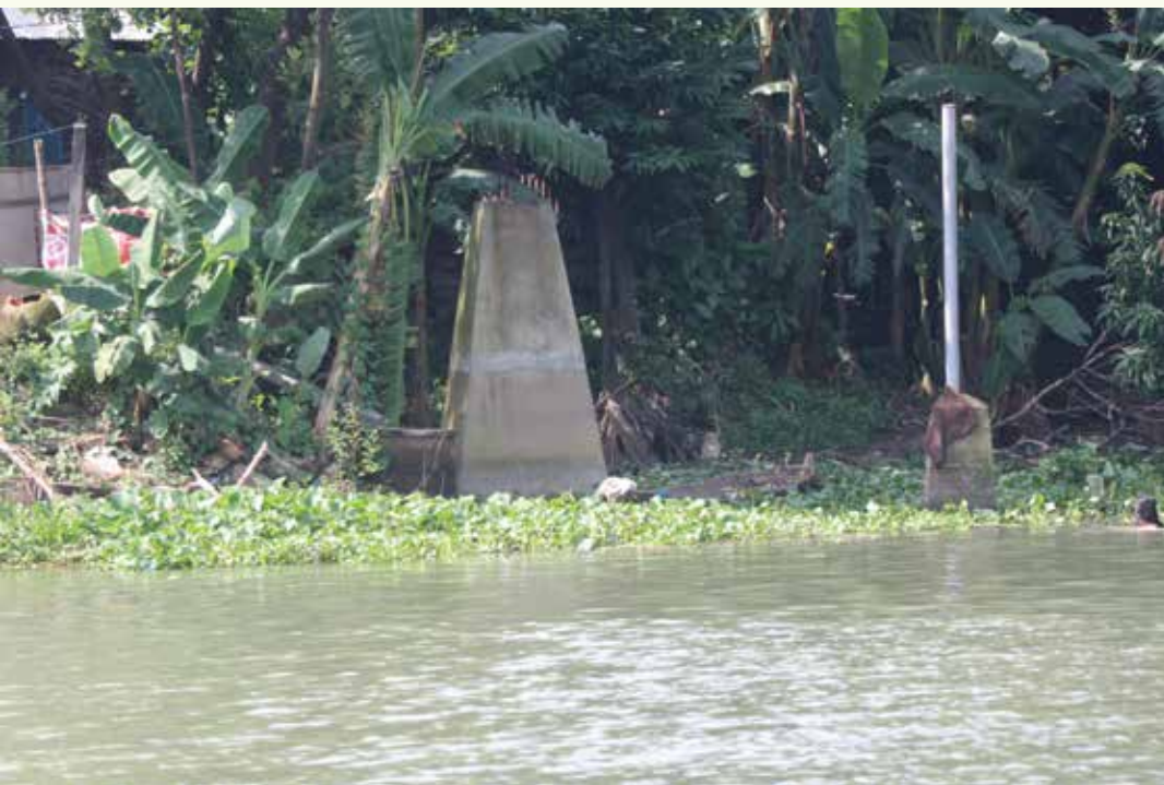
Photo: Faulty Pillars along Buriganga, East and West
